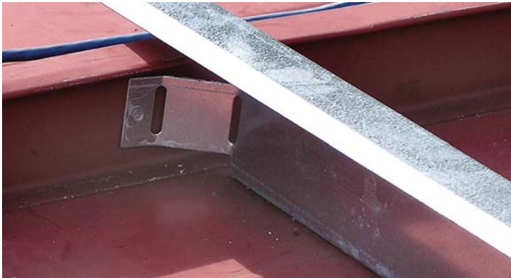
New Trapezoidal standing seam being installed over an old Vertical Rib standing seam with stand-off clips.
